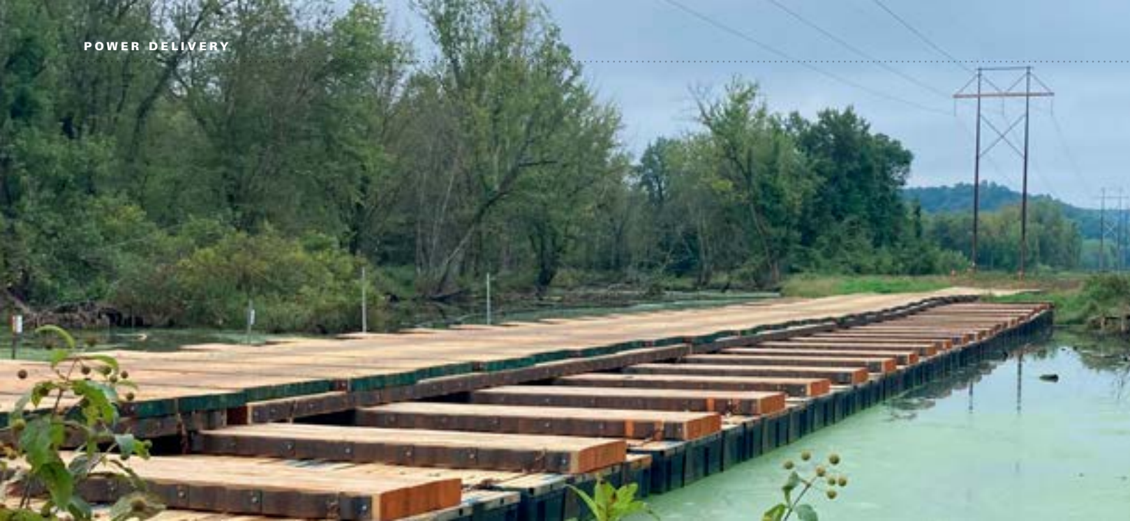
As part of the Badger Hollow Network Upgrades Project, we replaced a transmission structure on an island 400 feet into the Wisconsin River. Water levels in the floodplain of the region can vary, so the team chained four different types of mats together and anchored them to shore, creating a road across the river to support a 140,000-pound drill rig.
