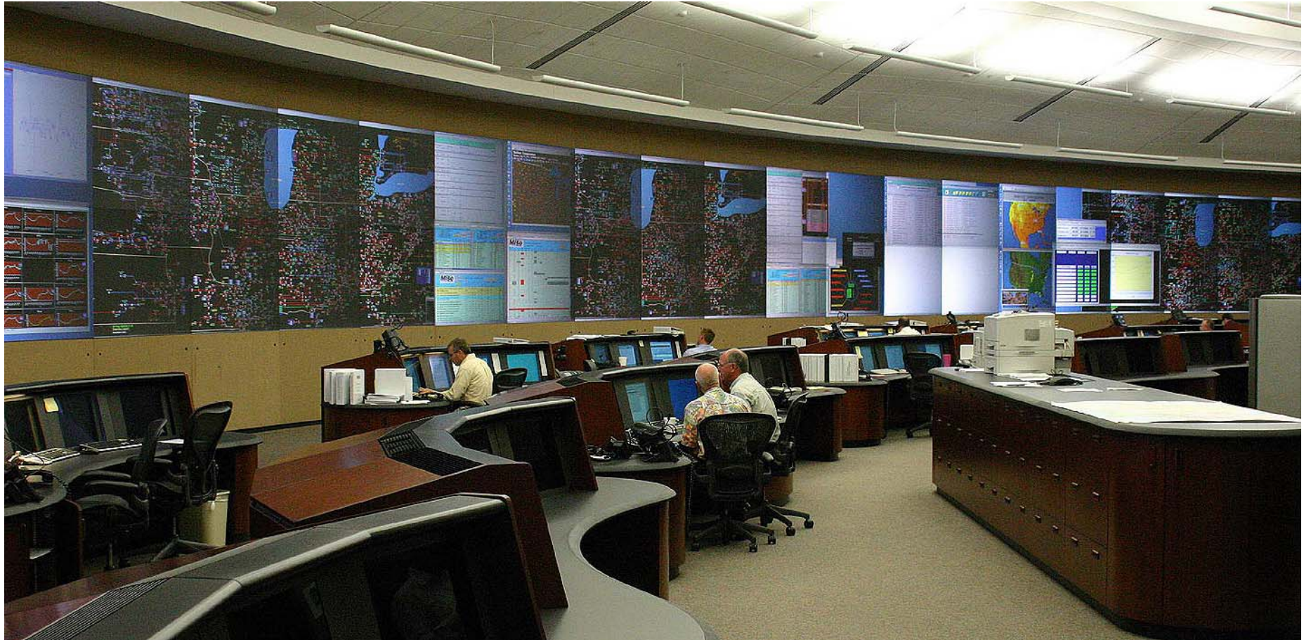
Midwest ISO Carmel Control Room
