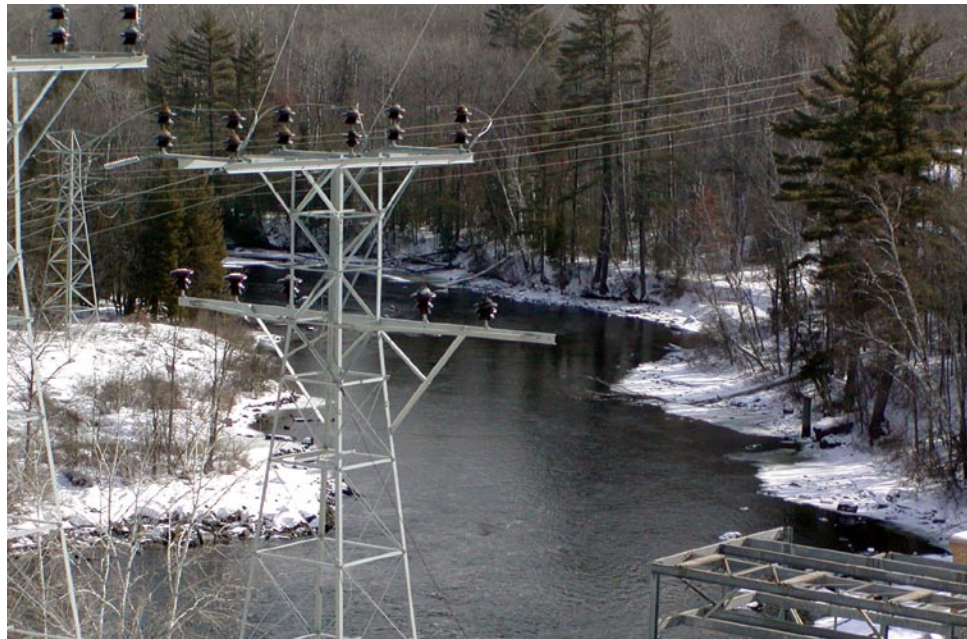
Part of ATC's proposal for Crivitz-High Falls included replacing aged structures such as this one.
