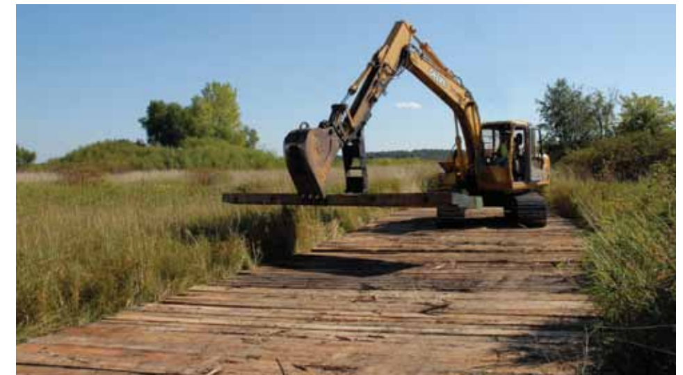
Matting equalizes the weight over an underground transmission line
